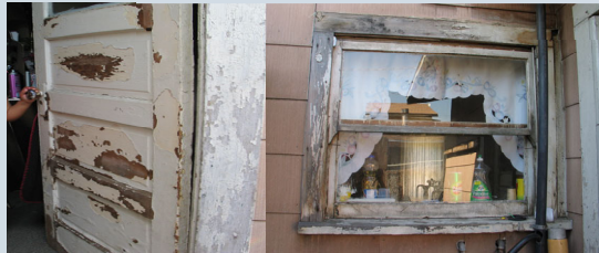
Paint in Homes Built Before 1978
